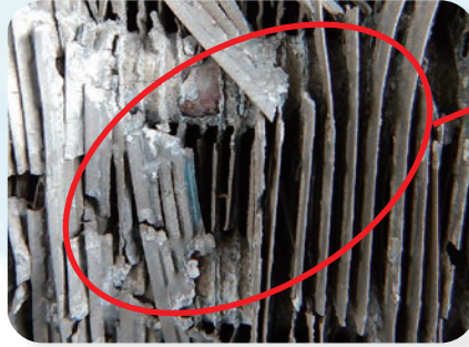
Inadequate Cooling Performance
