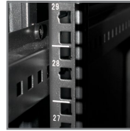
EQUIPMENT HEIGHT MEASUREMENT (U-MARK)
