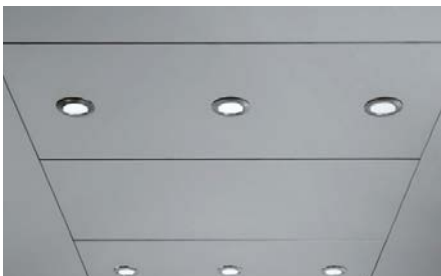
Ceiling lighting - standard LED round spot downlights*
